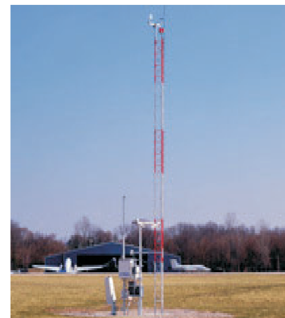
AWODS Sensor on a Mast
