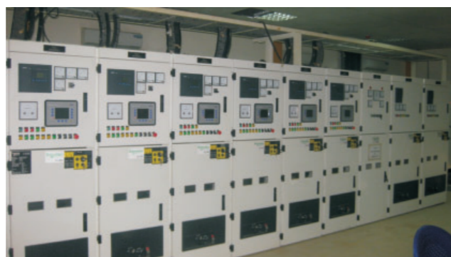
The brand new electrical switchboard master panels at the new powerhouse, May 2013
