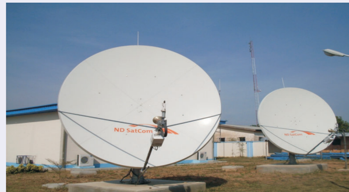
Two-node VSAT Hub at Kano ACC
