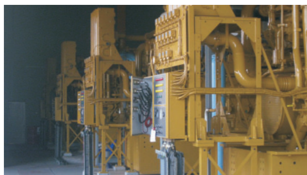
The new MMIA 4.85MVA generators, May 2013
