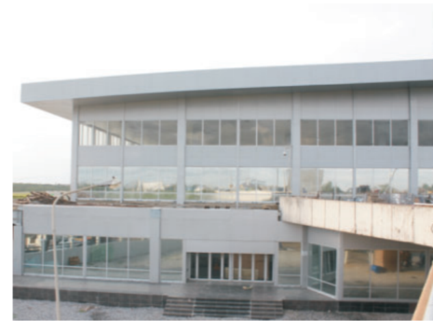
MMIA Expansion and Upgrade Project- the nearly completed 'E' Wing Extension, May 2013, which together with the 'D' extension, will ease the bottlenecks at MMA, adding much needed capacity to meet demand while changing the passenger experience into a positive one.
