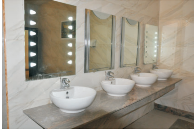
Newly remodelled MAKIA toilet facilities
