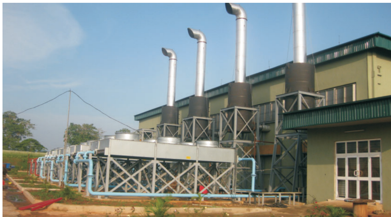
The new MMIA electrical power plant, May 2013
