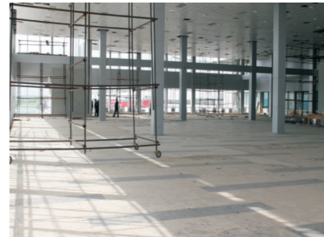
The new 'E' departures Immigration and security screening hall awaiting the installation of immigration counters and FAAN's new security screening equipment
